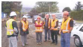
Trustees view the new VSS site along with Superintendent Rundell and Stuart Kamstra, Project Co-ordinator
